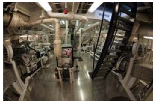
Delta Cathryn's yacht-white engine room holds two Cat 3516C main engines delivering almost 6,800 hp to the tug's Rolls-Royce z-drives. The boat's 40-foot beam and deep skeg add to its braking power. (Alan Haig-Brown photo)
